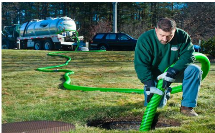
Figure 5: Vacuum truck cleaning of gravity grease interceptor
