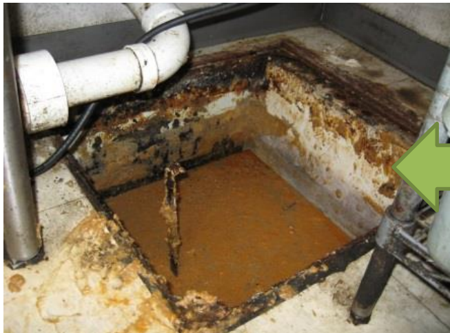
Scrape side and inspect baffles and flow restrictors
