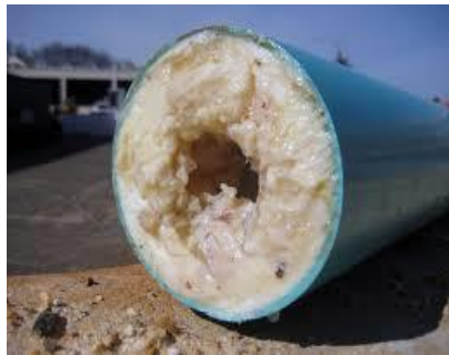
Figure 1: Image of FOG in pipe
