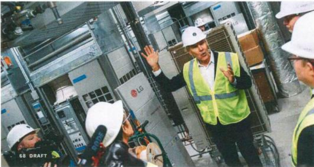
High-efficiency HVAC system in the Berkman in downtown Rochester, one of many sustainability features that earned the building Silver LEED certification from the U.S. Green Building Council.
