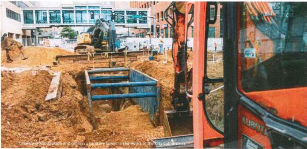
Construction to impact and install a sanitary sewer in the Heart of the City sub-district.
