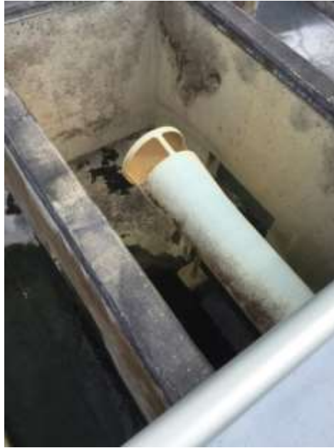
Figure 2-9. Chlorine mixing tube at chlorine contact inlet
