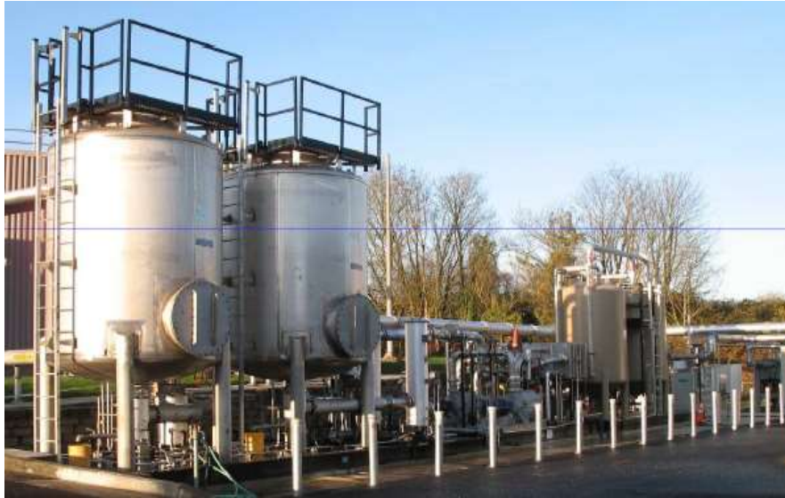
Figure 2-2. DG treatment system, Columbia Boulevard WWTP
