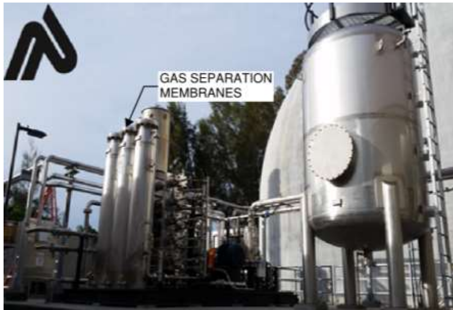
Figure 2-5. DG upgrading system at San Mateo WWTP (California) using Unison's BioCNG system Includes H 2 S removal, moisture removal, compression, siloxane removal, and membrane separation.
