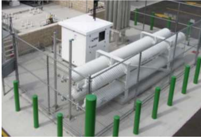
Figure 2-10. High-pressure CNG storage bank for on-site vehicle fueling
