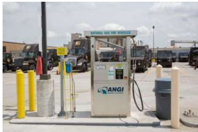
Figure 2-11. On-site vehicle fueling dispenser
