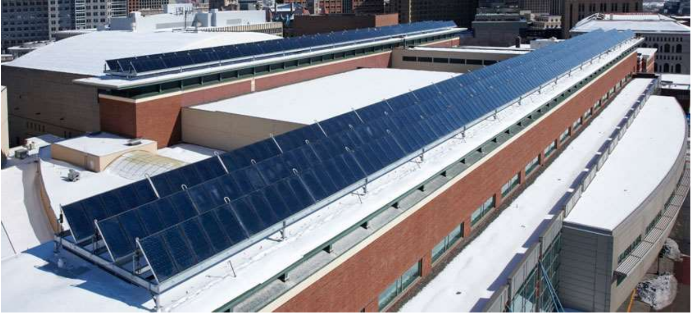
Figure 2-1. 1.5 MW thermal hot water solar system on roof of St. Paul RiverCentre
