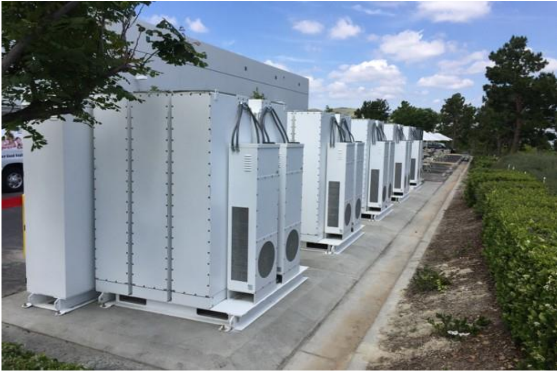
Figure 3-7: Tesla (3) 1MW / 2MWh Batteries
