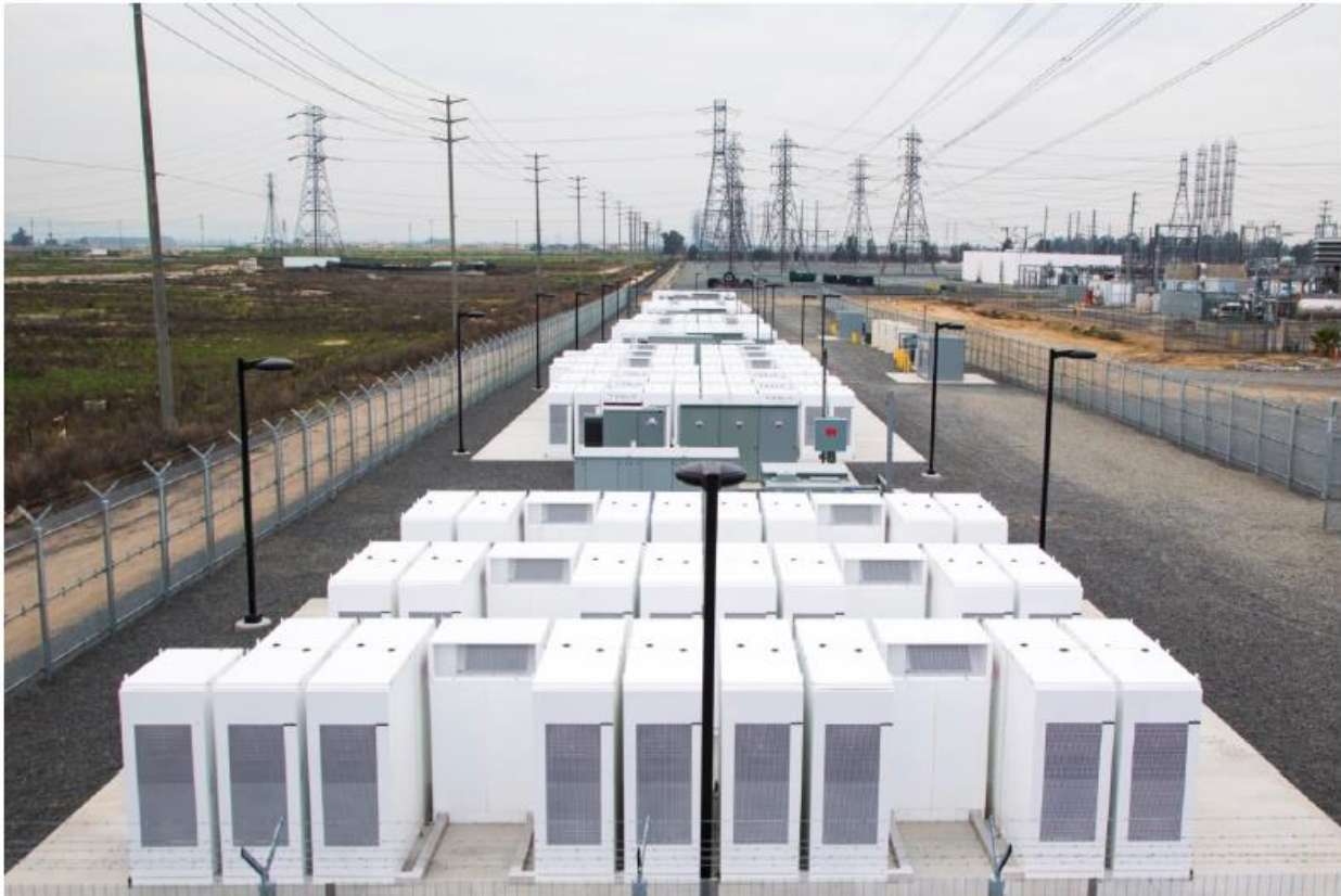
Figure 3-8: Southern California Edison 20MW/ 80 MWh
