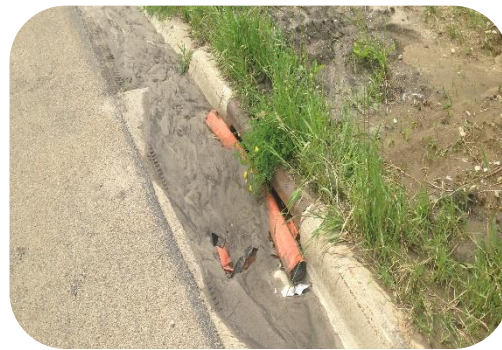
Inlet Protection Violation
