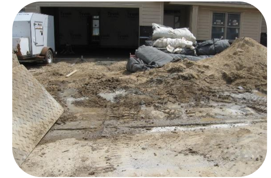
Construction Site Entrance - Violation
