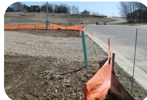
Construction Site Entrance - Compliance
