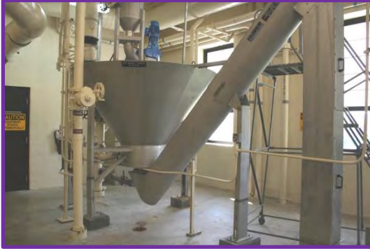
Grit Washing Process
