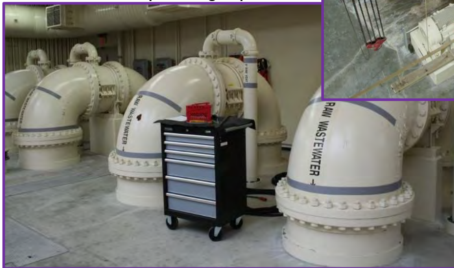
Raw Wastewater Pump Discharge Pipes
