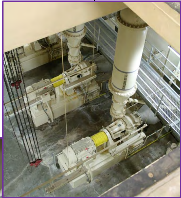
Raw Wastewater Pump Entrance Station
