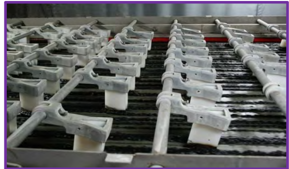
Gravity Belt Sludge Thickener
