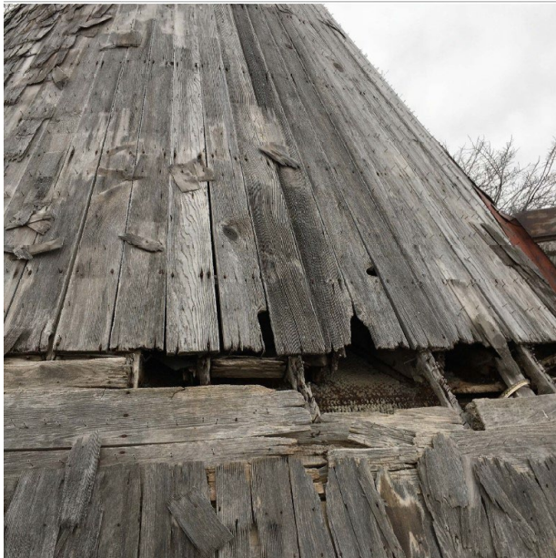
Deterioration at roof.
