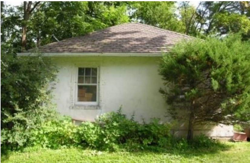
Stucco wall and brick veneer detailing at garage's south façade, looking north
