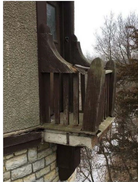
Deterioration at balcony
