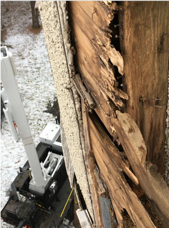
Existing condition of the stucco.
