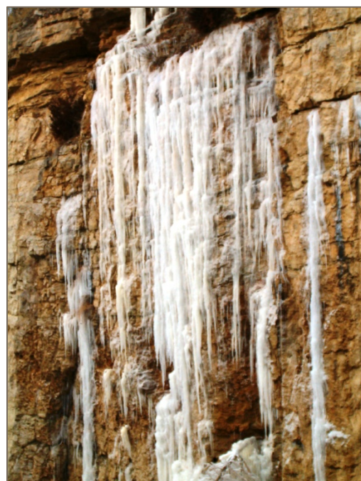
Groundwater flow freezes when exposed at area road cuts.
